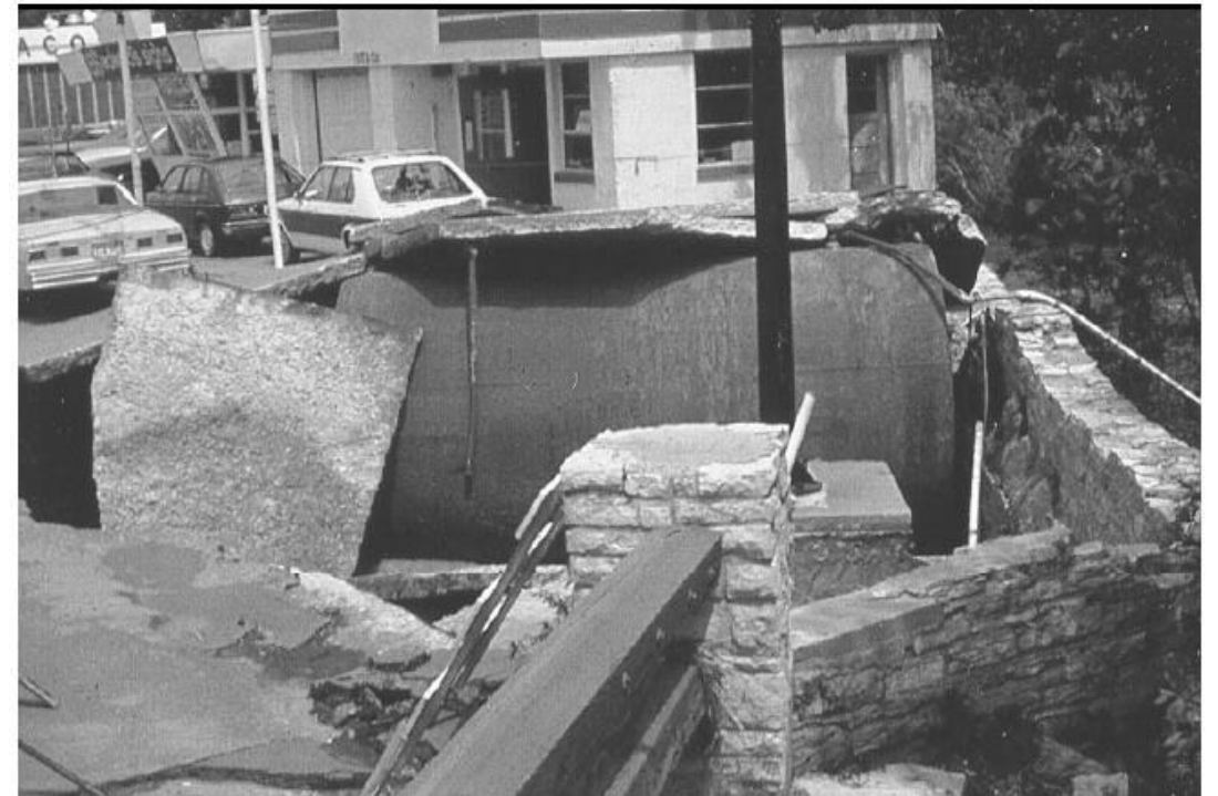
UST lifted by buoyant force
